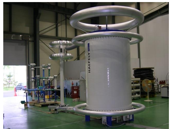
A System with 300 kV test transformer and HV divider
