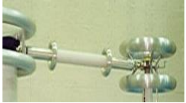
Typical damping resistor arrangement on a 300 kV system
